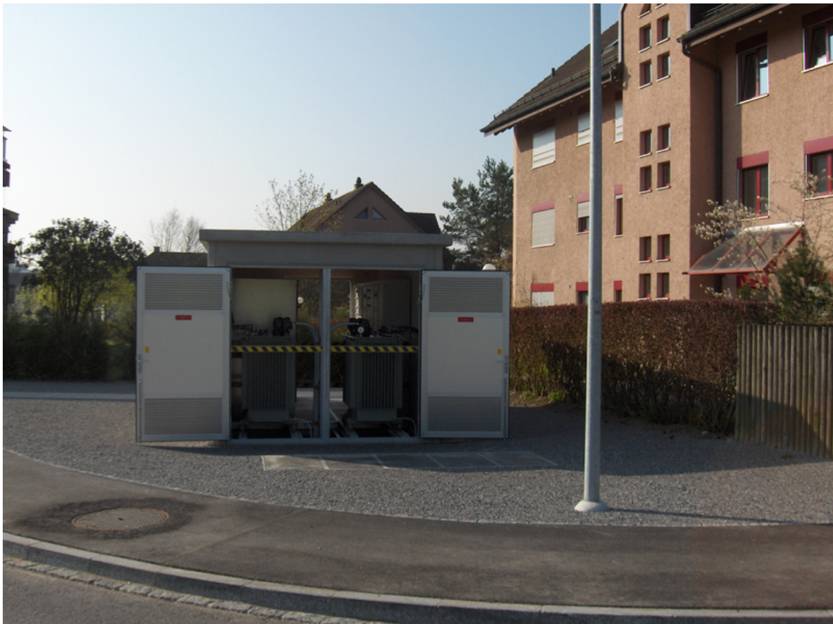
Neue Trafostation "Hürdli"
